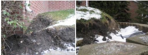
Redesign and excavate for better drainage away from structures – revise downspout design layout. Hire professional to design as necessary.
